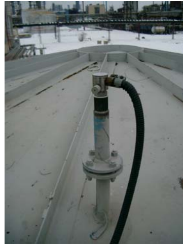
Ultrasonic level sensor of upper loading of sulfuric acid
