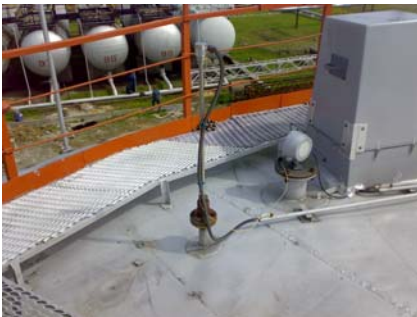
Ultrasonic Level Sensor on the reservoir of Komsomolskogo-na-Amure Oil Refining Plant
