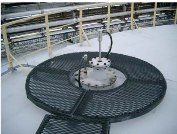
Non-contact level measuring device and ultrasonic
