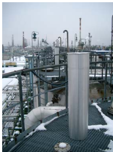
Set of measuring devices covered with protective housing
