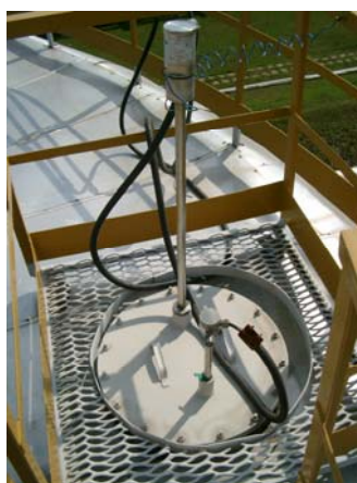
Operation stations of the level control and pump work system
