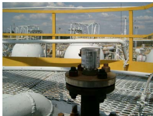
Ultrasonic level Sensor on the reservoir with liquefied butane
